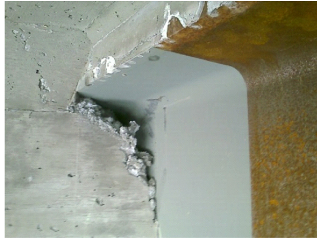
Figure 14 Badly Consolidated Concrete
