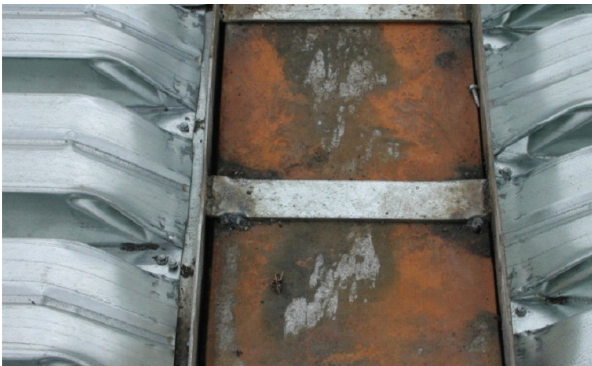
Figure 3 Steel SIP Forms Incorrectly Installed
