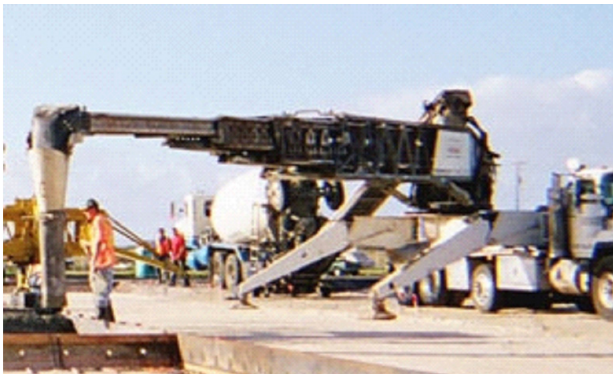
Figure 9 Conveyor with Trunk
