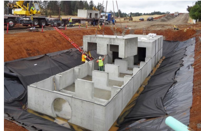
Figure B.4 Concrete Stormwater Vault
