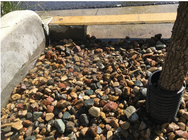
Figure 4.8 Before – SCM Constructed at the Incorrect Elevations
