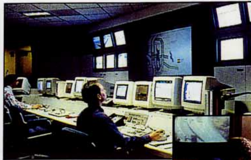
Traffic Operations Center
